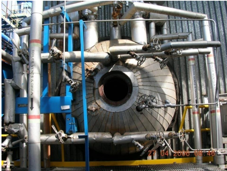
Steam drum of a boiler power plant
