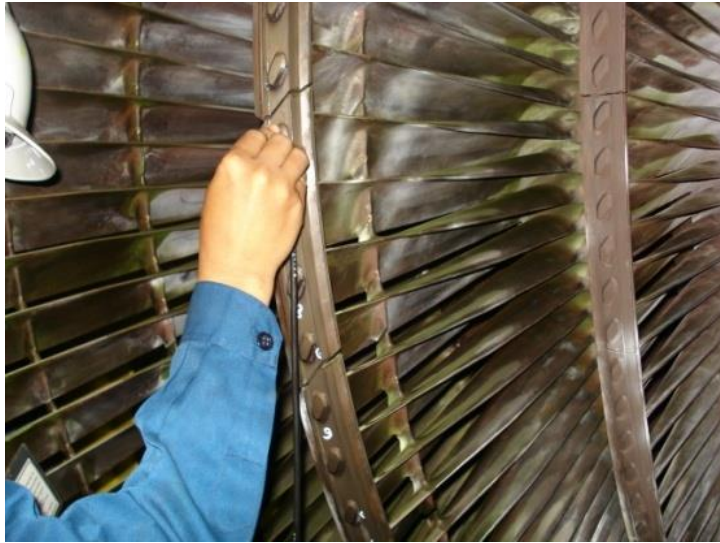
Steam Turbine Rotor and Blades
