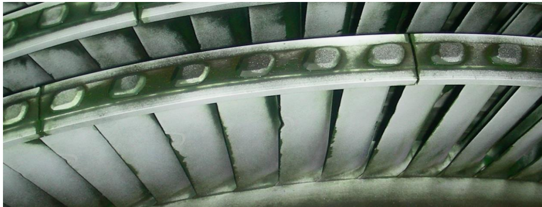
Erosion on trailing edge stage 12, shroud 3 blade no.5 , 6 and shroud 4 blades 1 to 6 (HP/Governor Side)
