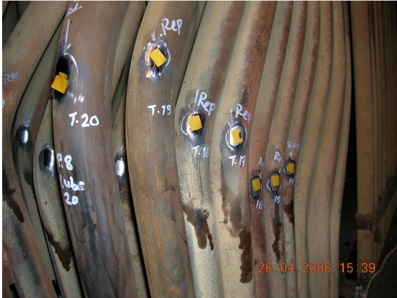
Replication test performed on several reheater boiler tubes.
