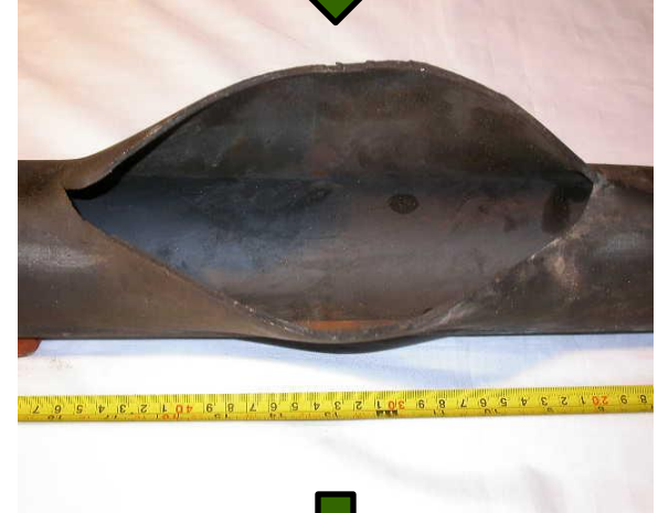
A ruptured boiler tube due to short term overheating
