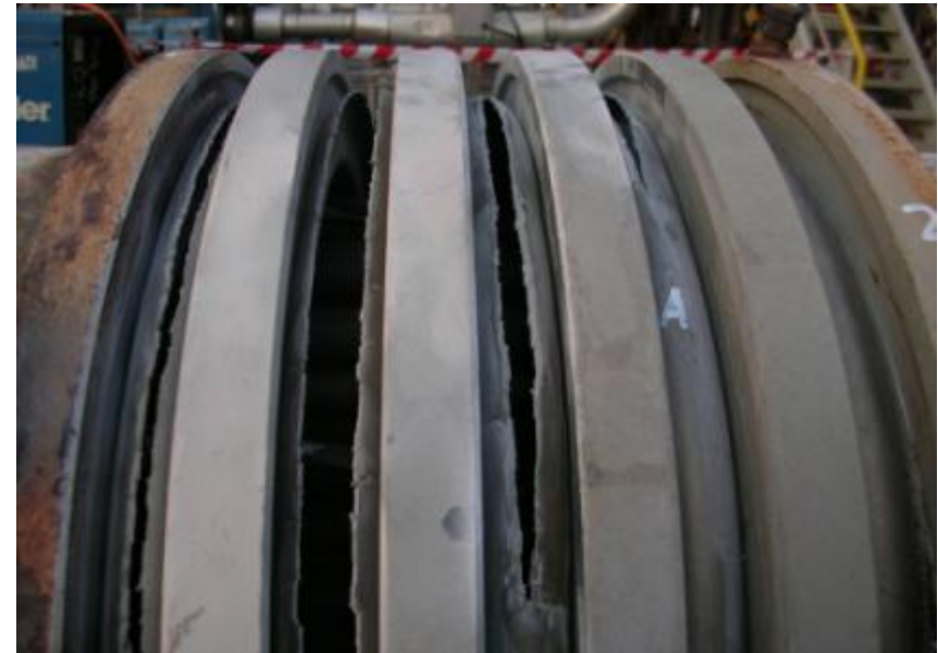
Close up view of a ruptured expansion bellows
