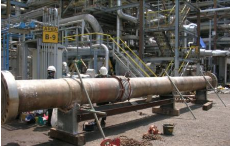
Photograph of a Pre-Heater equipped with an expansion bellows
